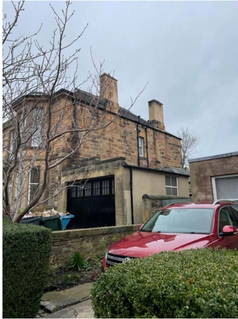
Figure 2 - Image shows the first floor side window that is to be replaced.
