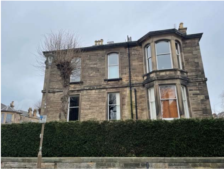
Figure 3 - Villa at corner of Glenorchy Terrace and Bright's Crescent. Top floor windows replaced with upvc.
