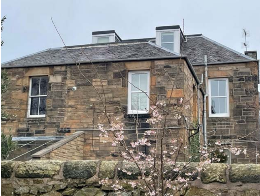
Figure 7 - View of UPVC windows to rear of 12 Mayfield Gardens. These can be seen from Glenorchy Terrace between the villas.
